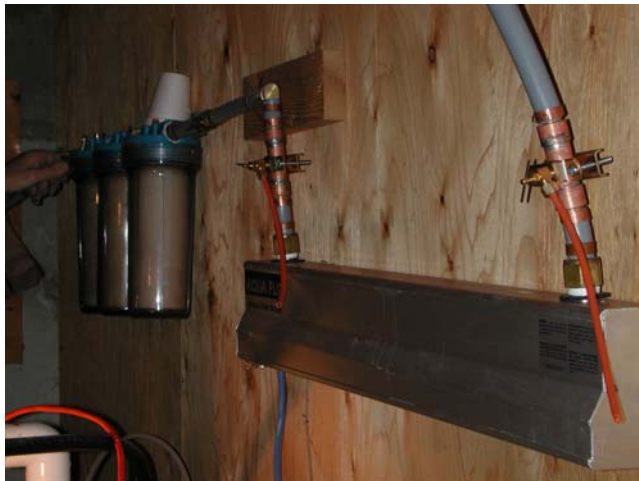
Figure 9: UV unit and cartridge pre-filters securely mounted to wall
